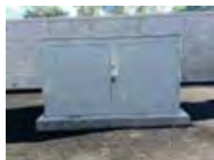
INDICATIVE PRIMARY METERING CABINET
