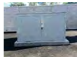
INDICATIVE PRIMARY METERING CABINET
